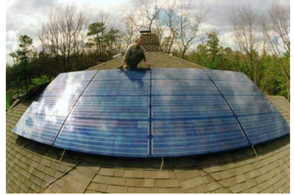
PHOTO FROM JERSEY SHORE SOLAR, NREL 09440
