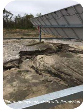
Photo: Strata Solar
